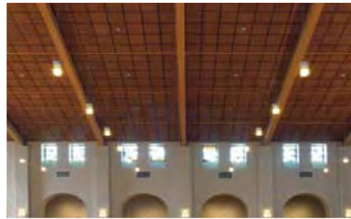
Inset: MetalWorks Tegular Extra Microperforated in Effects Cherry on Prelude® suspension system in Black; Mary Immaculate Catholic Church, Farmers Branch, TX
