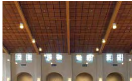
Inset: MetalWorks Tegular Extra Microperforated in Effects Cherry on Prelude® suspension system in Black; Mary Immaculate Catholic Church, Farmers Branch, TX
