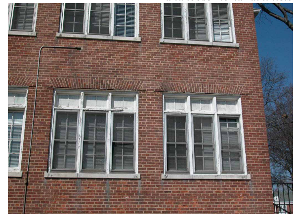
below: facade detail, H Building showing spalling brick and loose mortar at lintels
