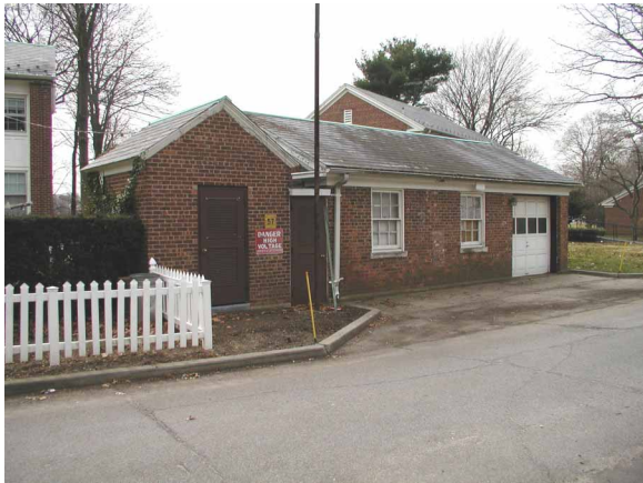
above: 5 kV Transformer Station on Quarters Service Road
