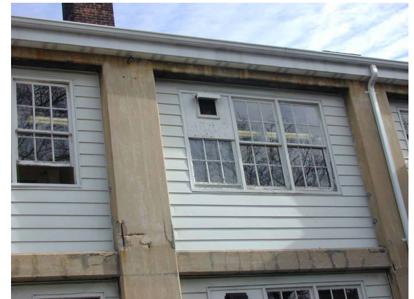
above: detail of rear of V Building showing spalling concrete and corroded reinforcing bar
