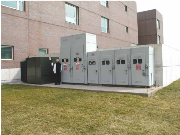
below: 13.8 kV Transformer and Switchgear at Building G
